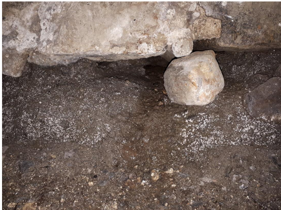
Figure 03 – Water infiltration and erosion under East foundation wall, adjacent to sump pit area.
