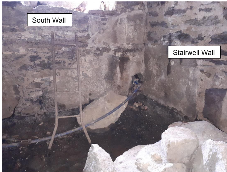
Figure 06 – Water infiltration underneath South foundation wall is evident, although exact location could not be established.
