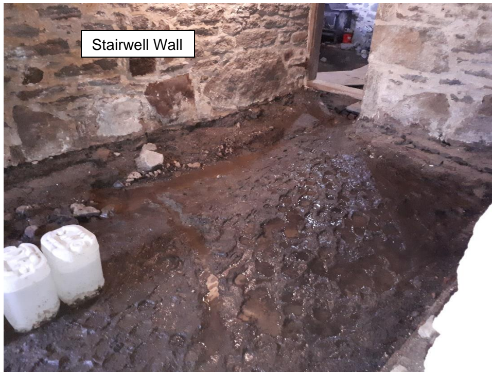
Figure 04 – Foundation segment adjacent to access stairs (interior view). Water accumulation on the floor. Drainage has been dug with slope towards sump pump.
