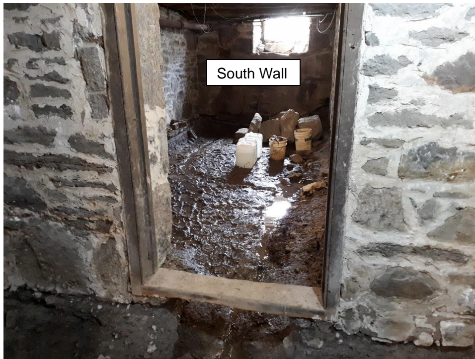
Figure 05 – Foundation segment adjacent to access stairs (exterior view). Water accumulation on the floor. Drainage has been dug with slope towards sump pump
