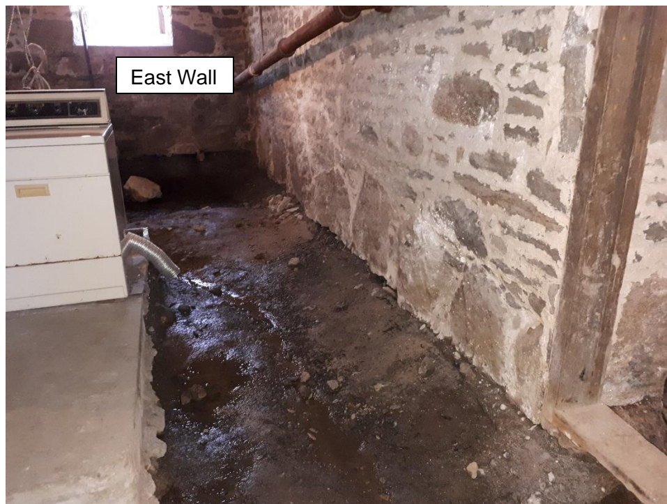
Figure 07 – Middle basement segment facing East wall. Water drainage path dug in floor, sloping to sump pump.
